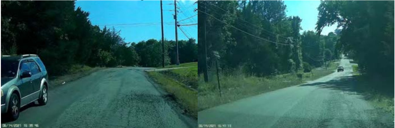
Above: Pavement Conditions Along Old Mayhew Road (Looking West)
